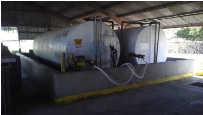
General view of the system
