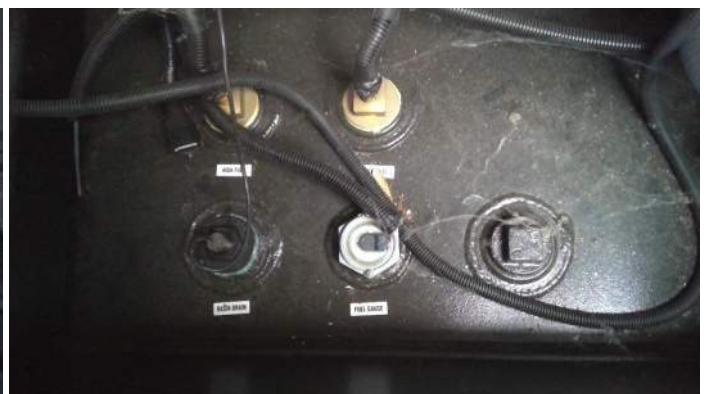
Overfill and leak sensors
