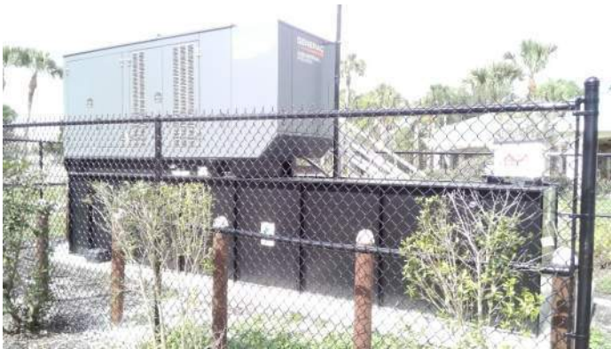
General view of the system
